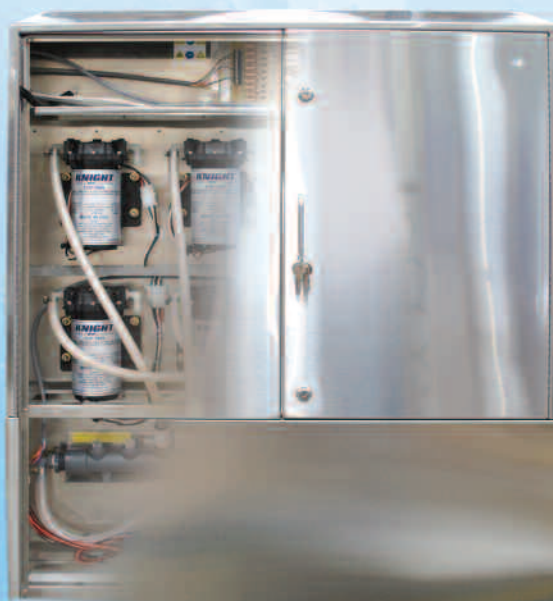
EDP Pump Cabinet
