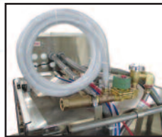
WATER CONNECTION POINT
